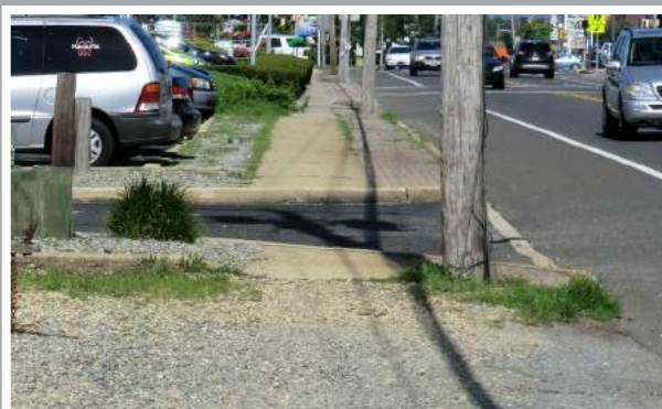
Wrong: Driveway cutting through sidewalk
