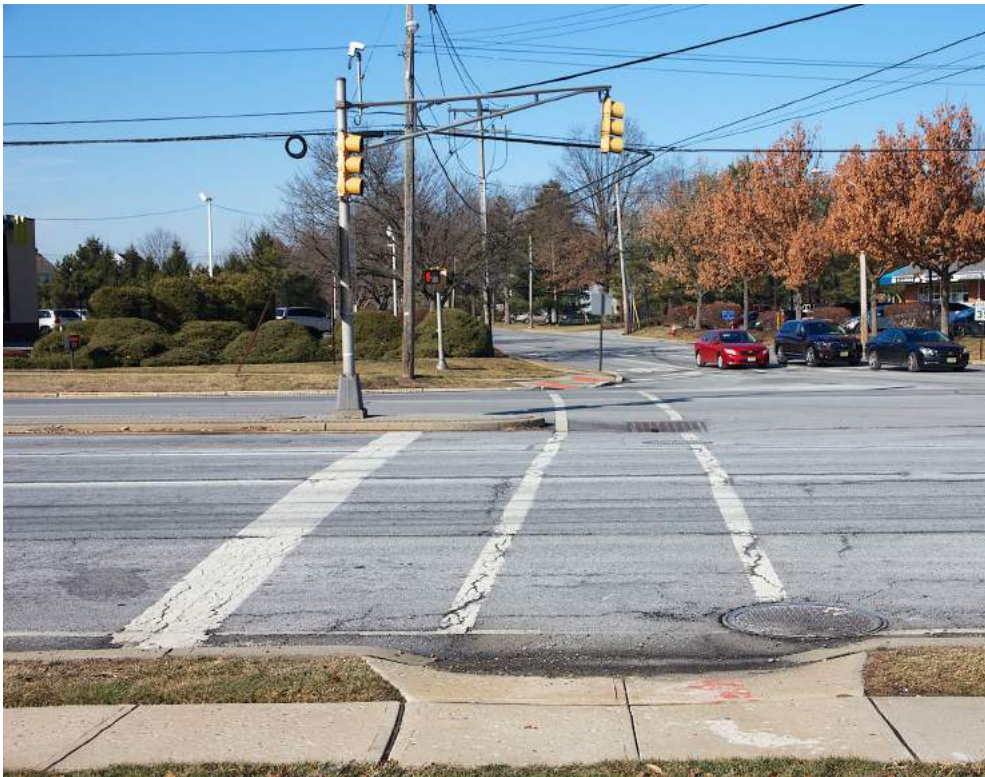
Worn detectable warning surface at SE corner, facing west
