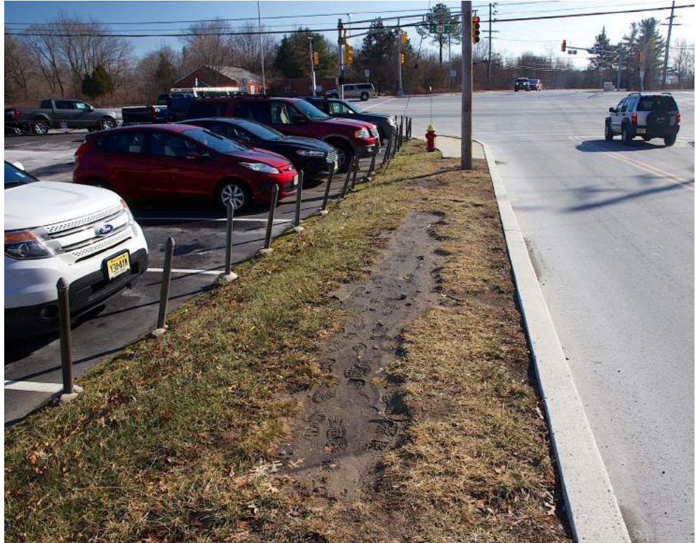
Worn path and utility obstruction along Hickory Corner Road near U.S. Route 130, facing east
